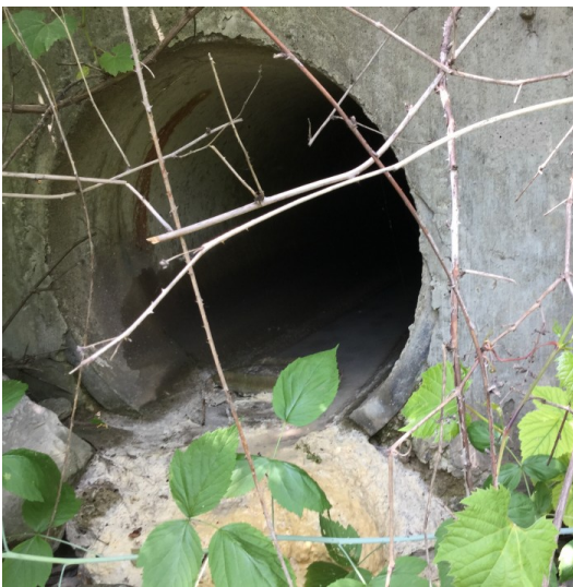
Stormwater Outfall from an Industrial Facility
