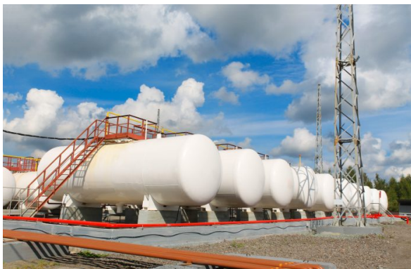
Aboveground Storage Tanks
