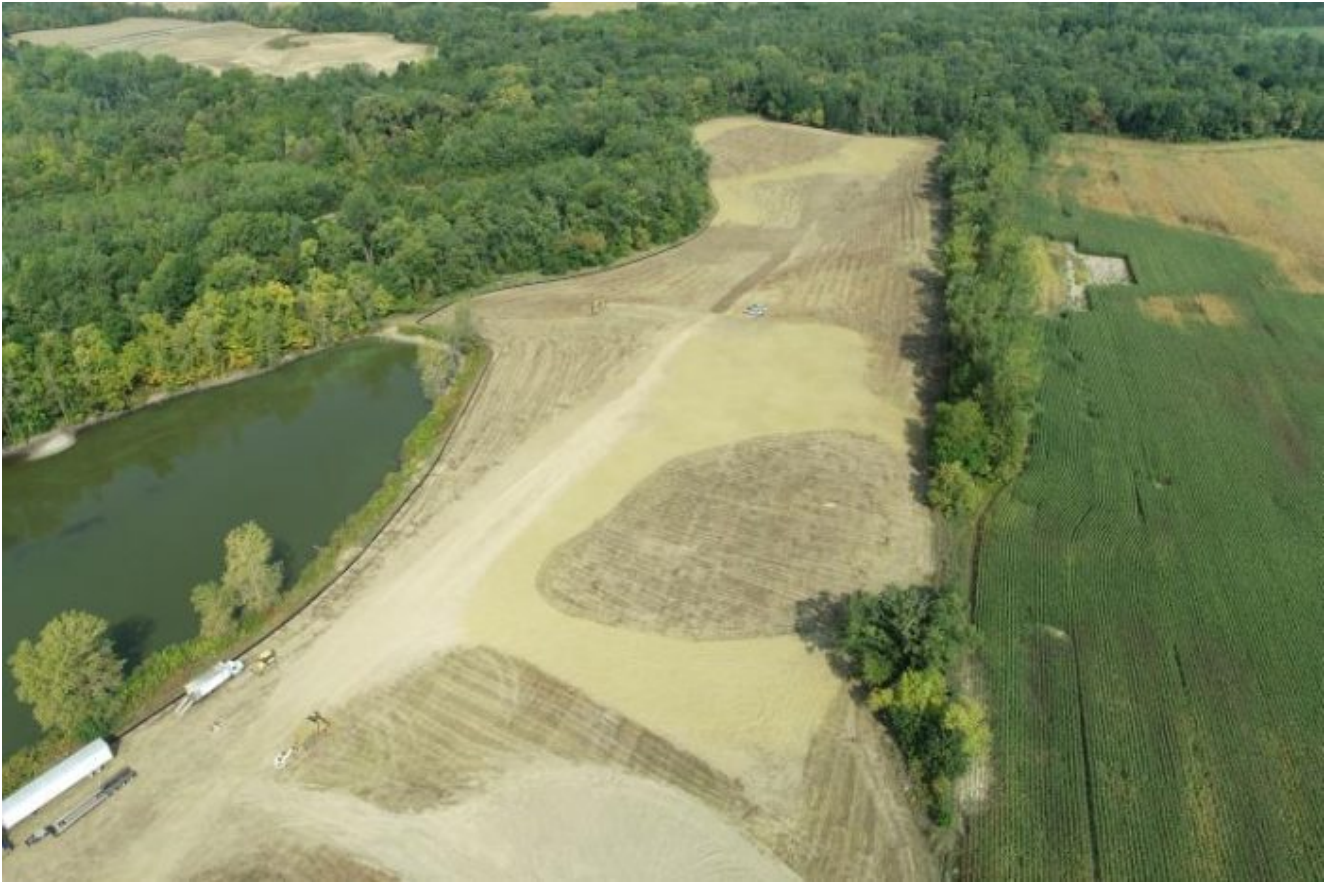
Agriculture field facing NW during construction (Drone image by EnviroScience, Jeff Niehaus)
